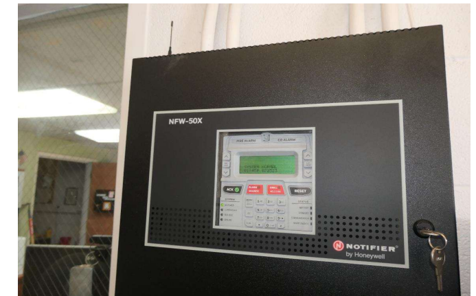
Fire alarm control panel
