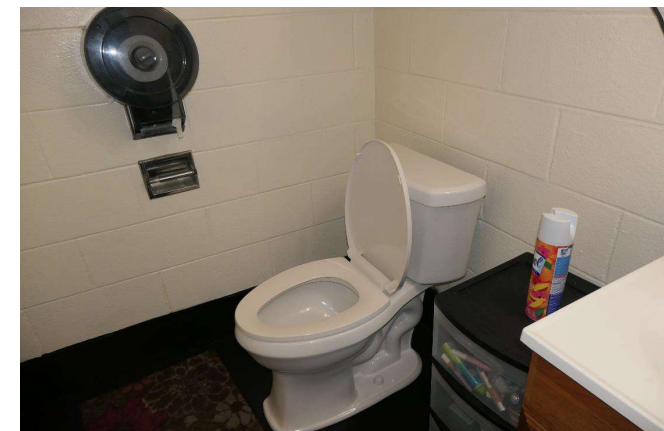
Interior bathroom finishes
