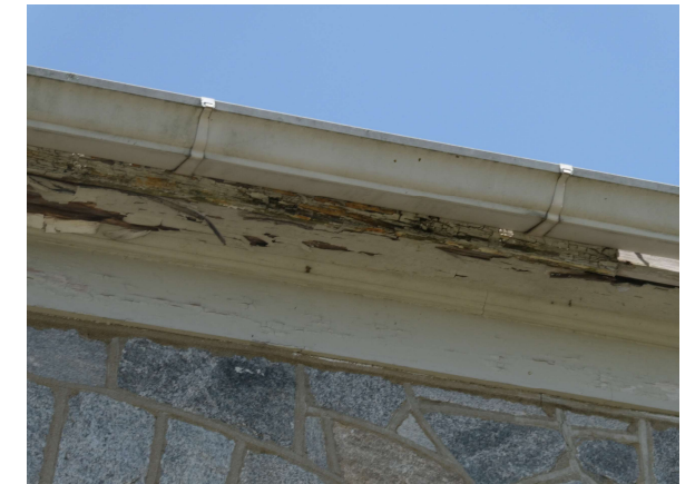
Damaged wood soffit under roof.
