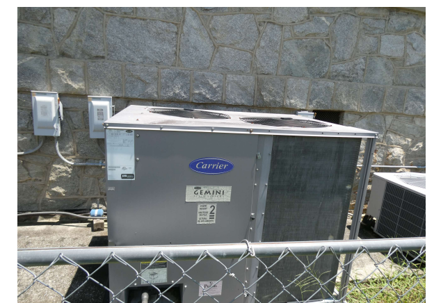
Split system air conditioning unit from 2013.
