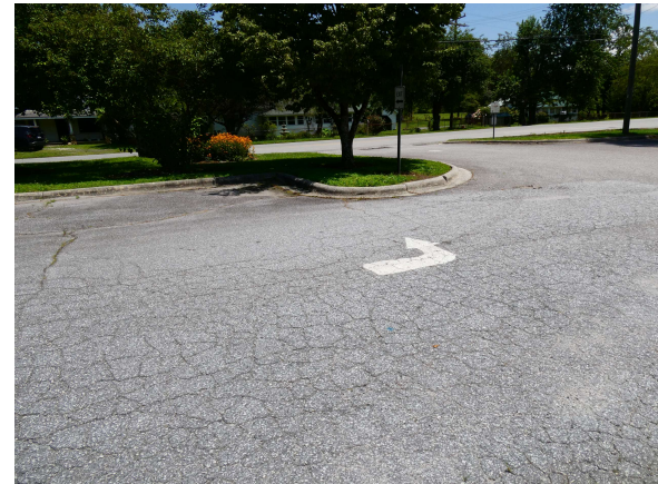
Alligator cracking of asphalt parking lot.
