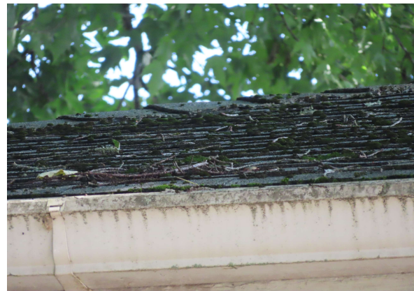
Organic growth at asphalt shingles.
