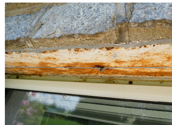
Corroded lintel at exterior windows.
