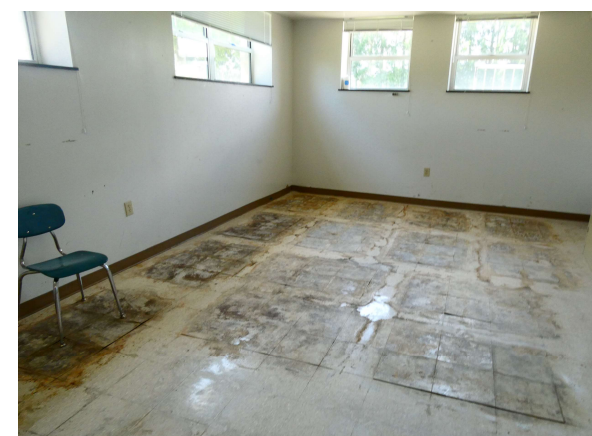
Deteriorated VCT flooring in basement floor.
