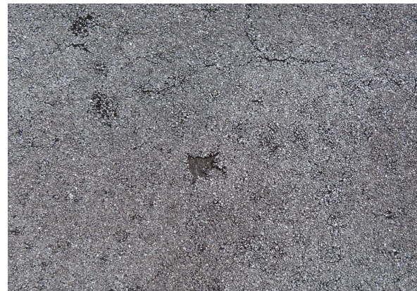
Deterioration of the built-up roof cap sheet.
