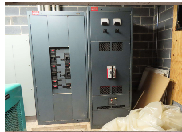
Obsolete electrical components, including main switch.
