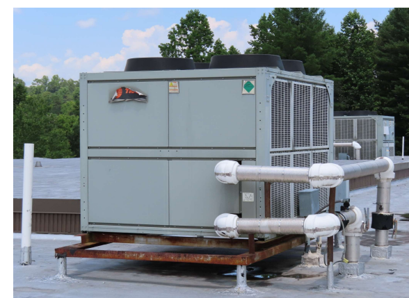
Typical air-cooled chiller.
