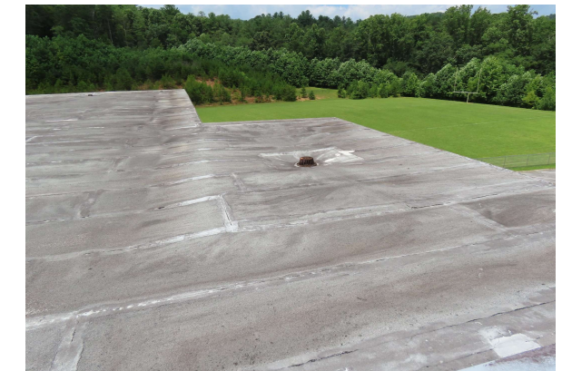
Failed seams noted at the built-up roof over the gym.
