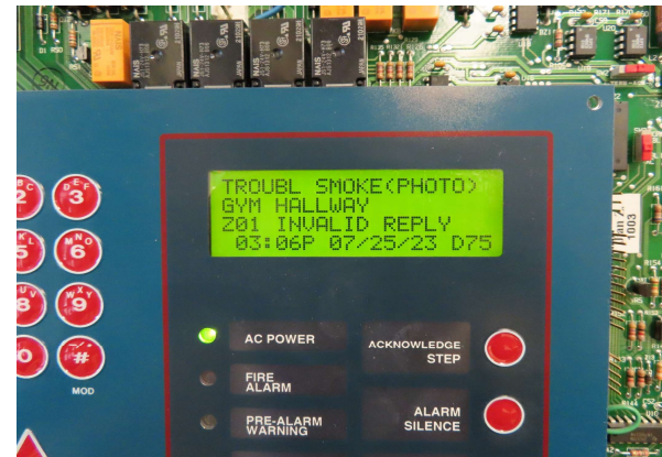
Obsolete fire alarm control panel with noted trouble alarms.
