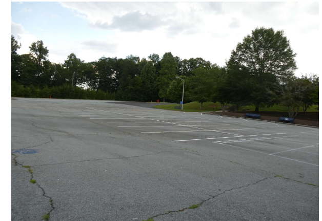
Asphalt parking lot with minor cracking.
