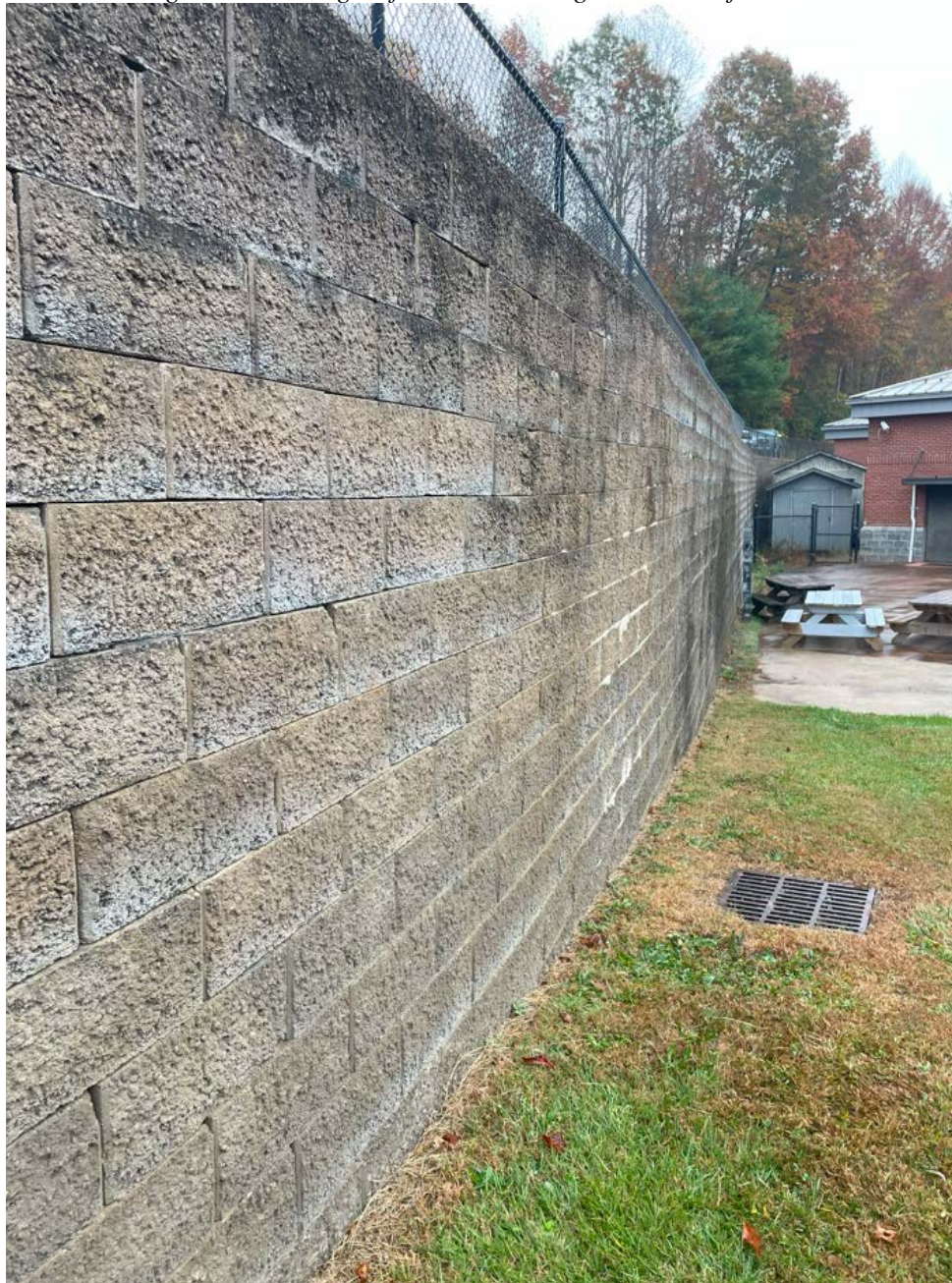
Figure 1: Existing Deflected Retaining Wall East of School
